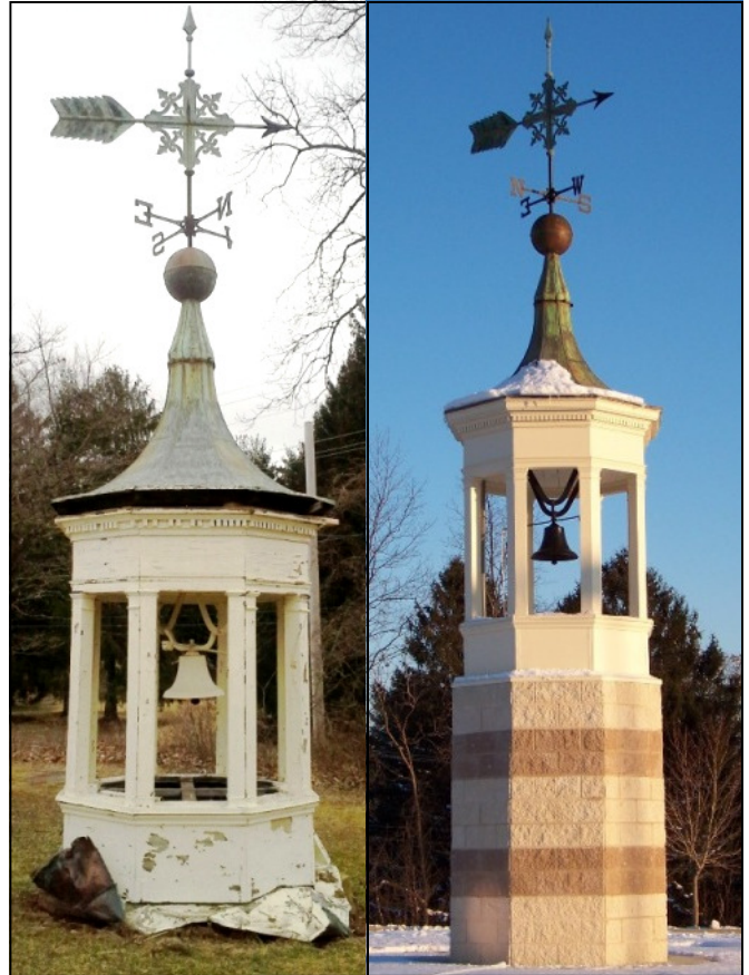
The cupola and its dramatic weathervane before and after its restoration by Roberson Preservation Services, Inc.
