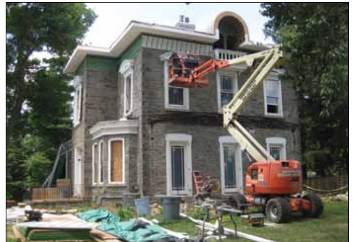
The windows on this building are being replaced with windows of an inappropriate type, pane configuration and possibly material.
