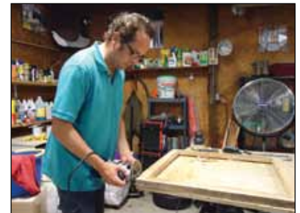
As part of a comprehensive restoration and energy upgrade, a homeowner routs his historic window sash to insert weather stripping.
