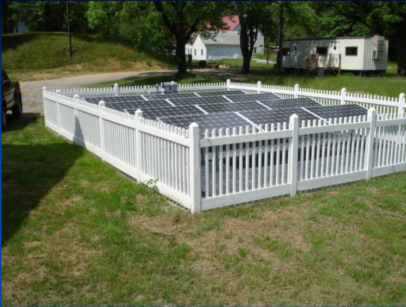
Freestanding Solar Panels in Rear Yard with Screening
