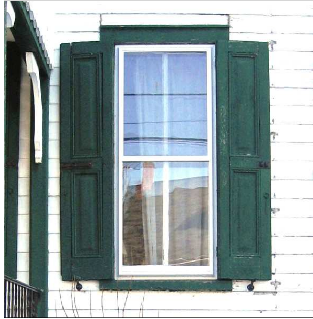
Storm windows can improve the efficiency of a window for less than the cost of replacing them, increasing R-value and reducing air infiltration.
